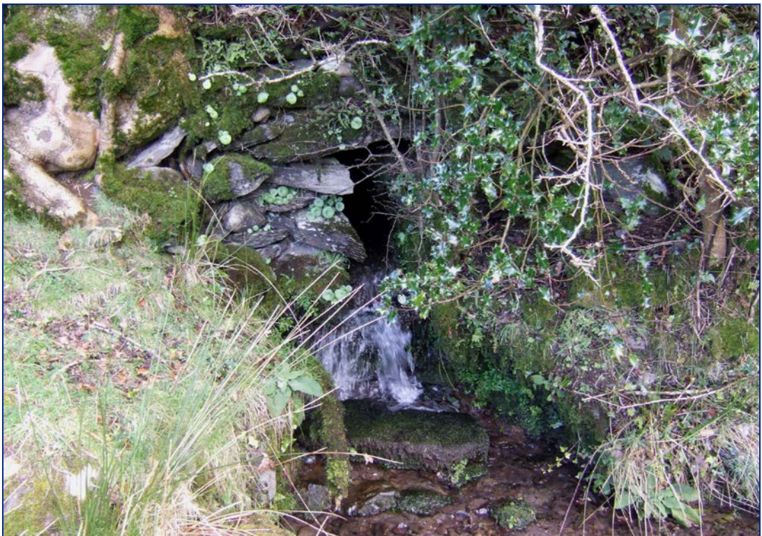
Figure 3.2: View of stone culvert in bank below N22. This will be covered by the proposed works.
