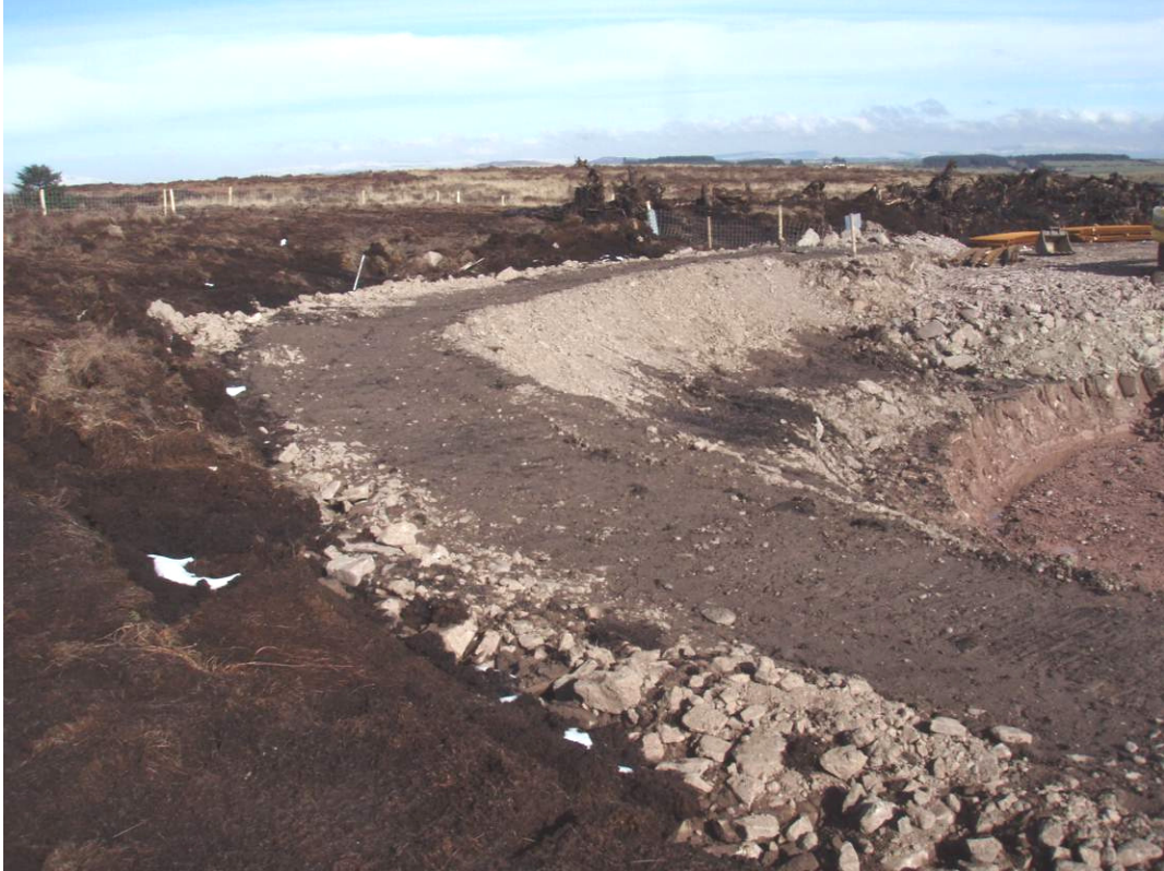
Figure 7-4 Rockfill berm around an area of deep peat on a previous ESB Wind Farm
